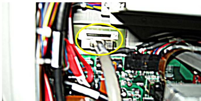
Figure 8-186 Boundary Scan cable connects BEP to Back Plane (BEP5 is illustrated)
