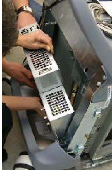
Figure 8-201 Main Power Supply installation
